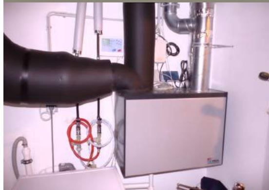
Air handling unit in utility room of a Certified Passive House
