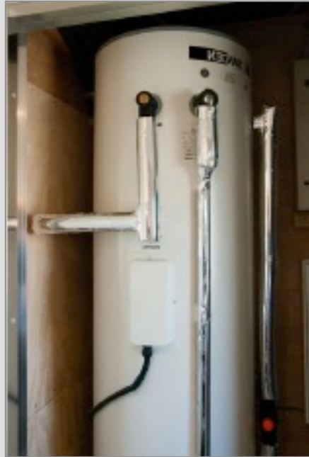
Sanden Heat Pump Domestic Hot water
