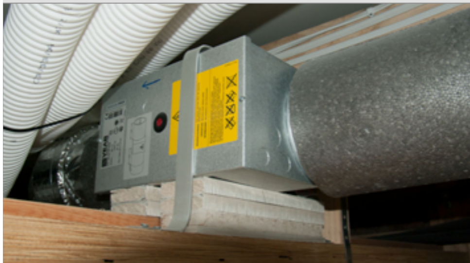
1.2 kW Electric Duct Heater
